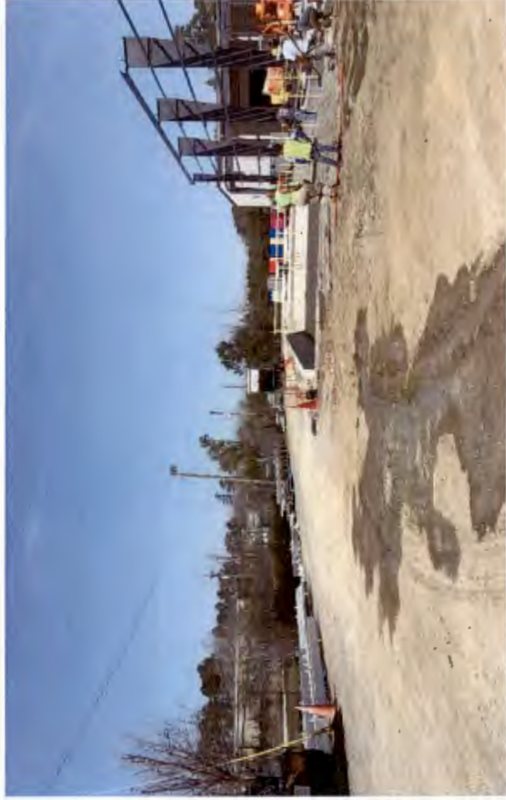
Loading dock encroachment
